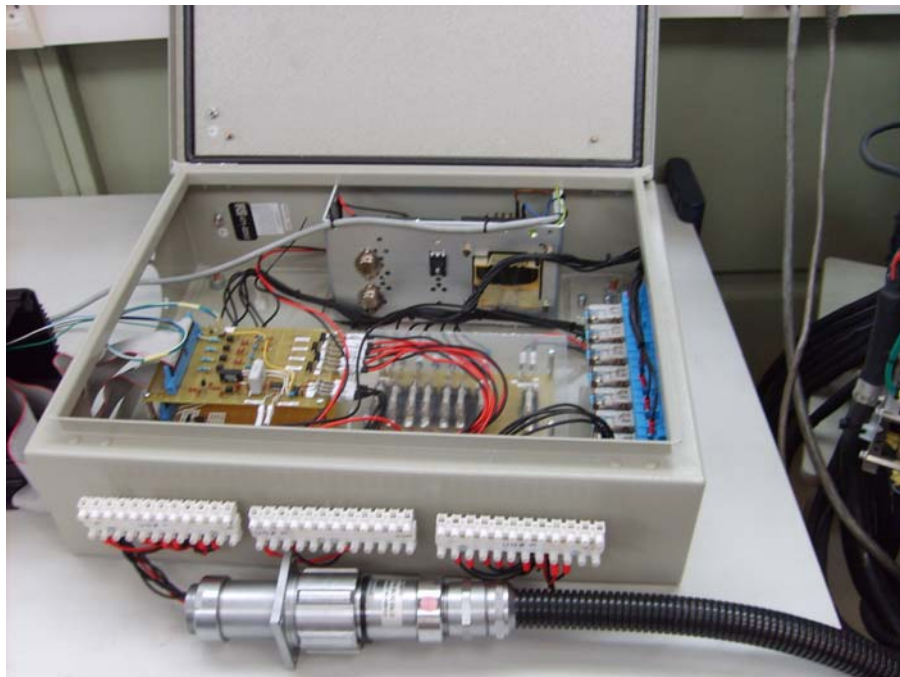
Figure 5. Photo of the electrical interface
